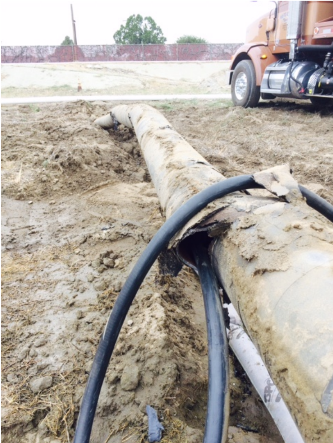
Photo 5: Facing north; Vacuum truck recovering residual liquids from the broken pipeline.
