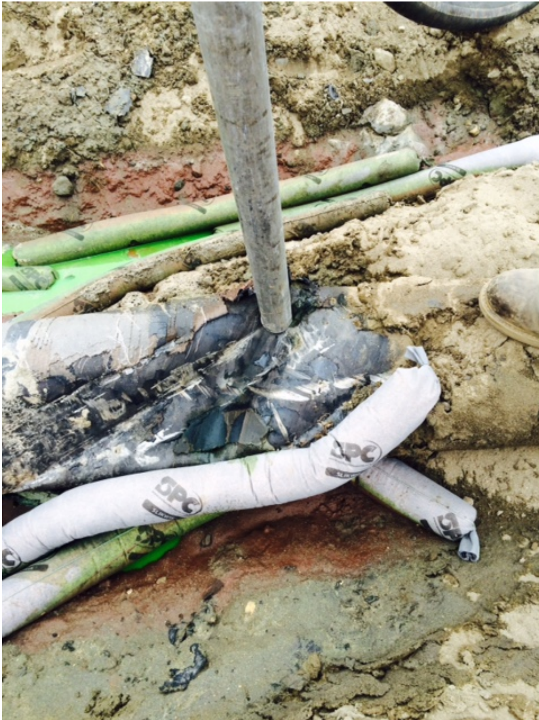
Photo 1: Vacuum truck recovering liquids directly from the damaged pipeline.
