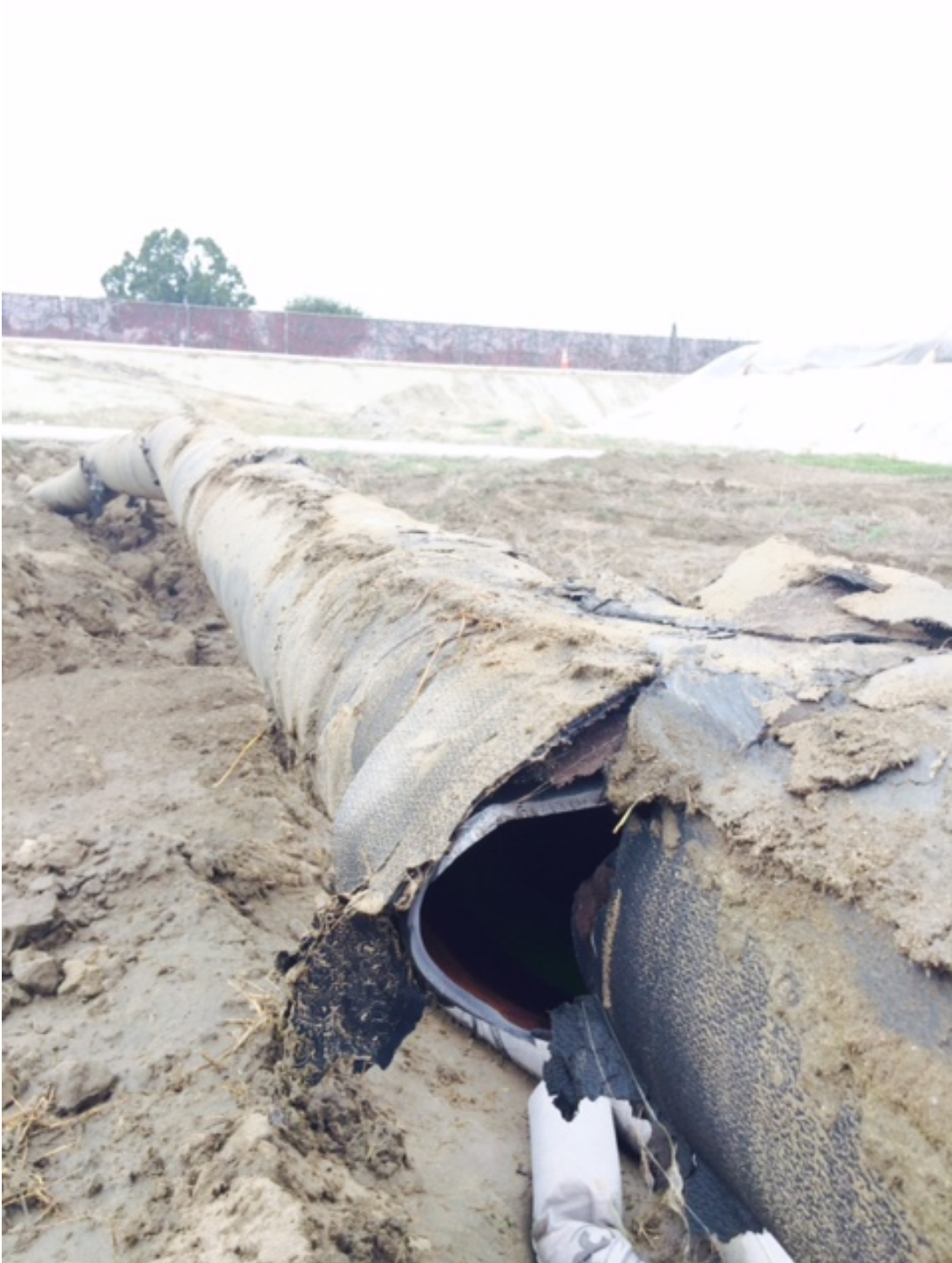
Photo 4: Facing north; Broken pipeline.
